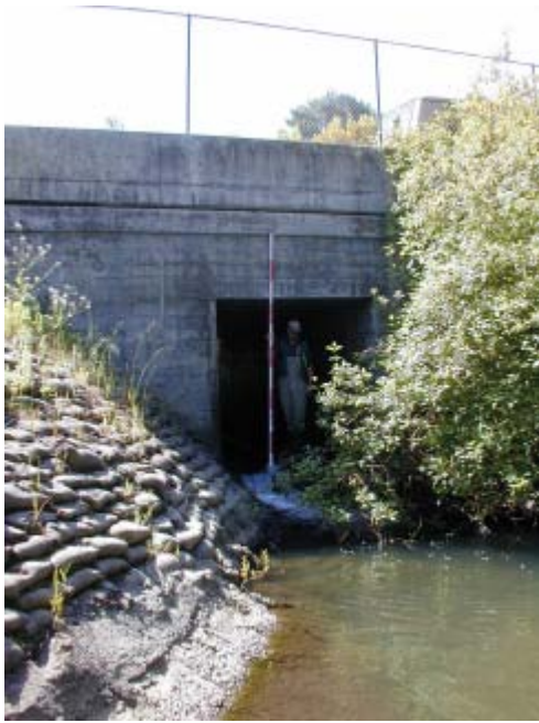
Adobe St Bridge on San Pedro Creek 5/28/03 Looking upstream at the culvert.
