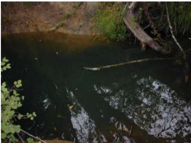
Edson Creek 7/10/03 Large scour pool just upstream of culvert inlet.
