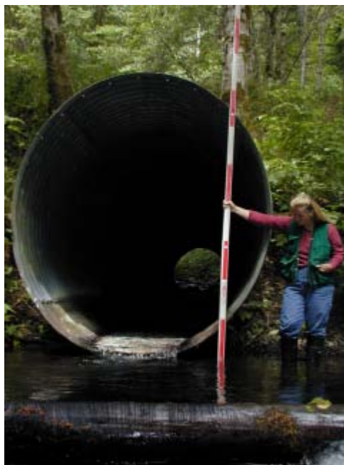
Fan Creek 7/15/03 Looking upstream at outlet. This culvert is not the one that will be replaced.
