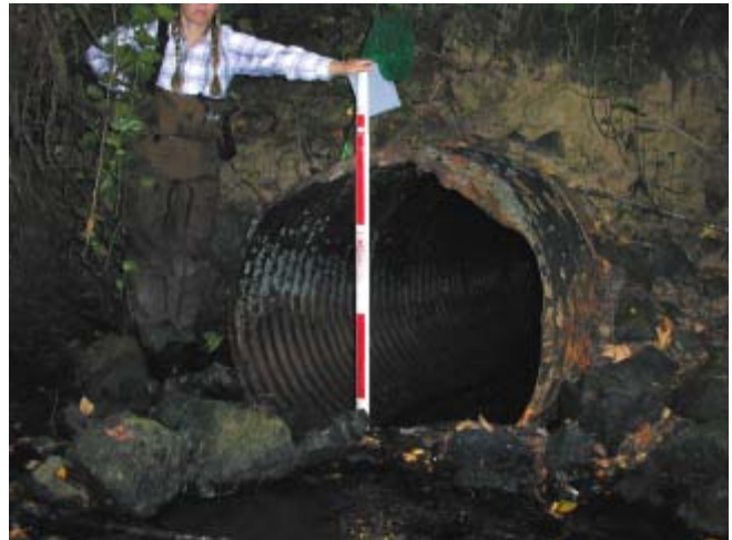
Hantz Creek 7/14/03 Looking downstream at pipe inlet with negative perch.
