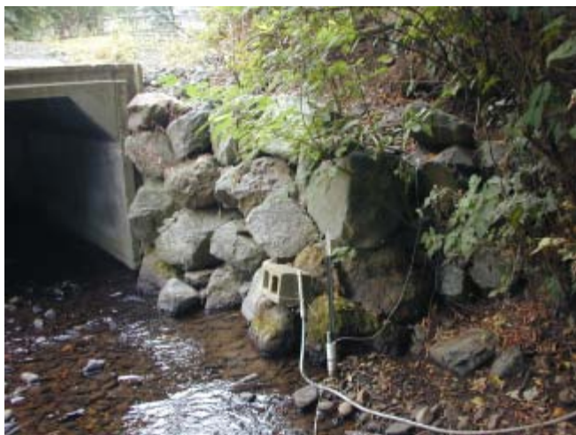
North Fork Newaukum Creek 8/11/03 Looking upstream at left bank of upper culvert.
