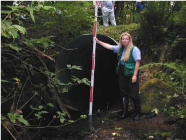
Cedar Creek 7/15/03 Looking downstream at inlet.
