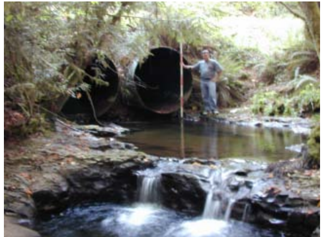
Oxbow Creek 9/ 2/03 Site of a culvert restoration that will occur soon. Culvert was identified using NFWF funds.
