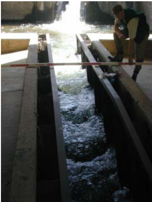
Capistrano St bridge San Pedro Creek 5/28/03 Close-up of fish ladder looking upstream.
