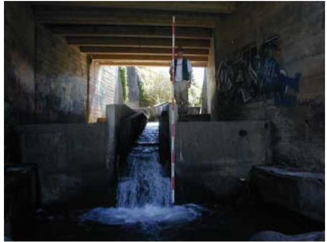
Capistrano St Bridge San Pedro Creek 5/28/03 Looking upstream at fish ladder underneath bridge.
