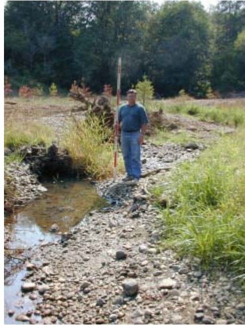
Green Creek 9/ 2/03 Stream meander restoration done downstream of the Green Creek culvert replacement.
