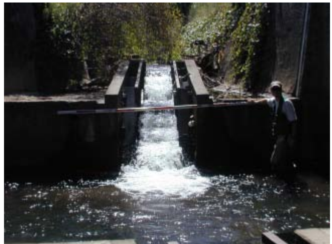
Capistrano St Bridge San Pedro Creek 5/28/03 Looking upstream at the upper fish ladder.
