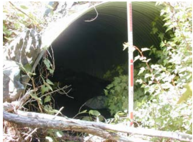
Taylor Creek 7/10/03 Looking downstream at inlet of overfilled culvert.
