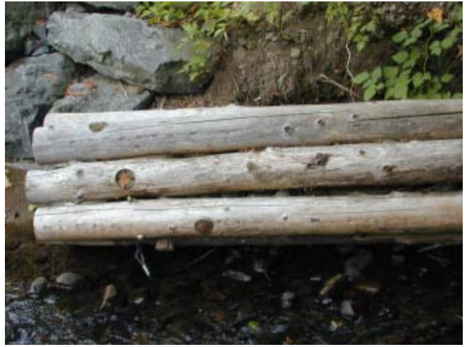
North Fork Newaukum Creek 8/11/03 L-log structure placed on the right bank just above the upper culvert inlet.
