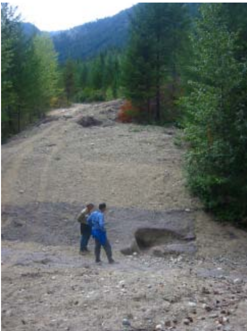
White River Floodplain 9/ 8/03 Kurt Beardslee and Gordon Congdon looking at sinkhole where the stream found an old culvert.
