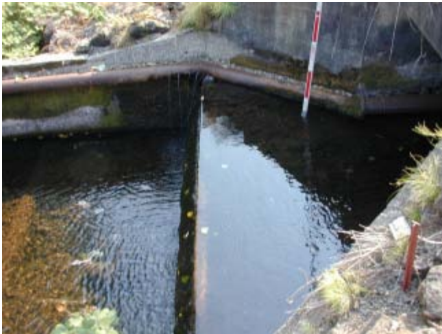
Stringer Creek 9/ 2/03 Site of a proposed fish passage restoration project. The project fell through when the landowners requested $30,000 in order to allow the project.
