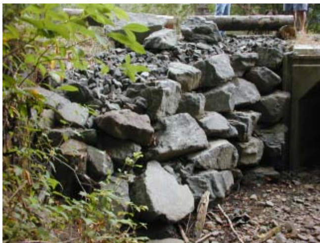
North Fork Newaukum Creek 8/11/03 Looking upstream at lower bank of upper culvert.
