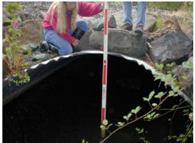
Squaw Creek 7/10/03 Looking downstream at culvert inlet. There were a series of three culverts on Squaw Creek that were replaced.
