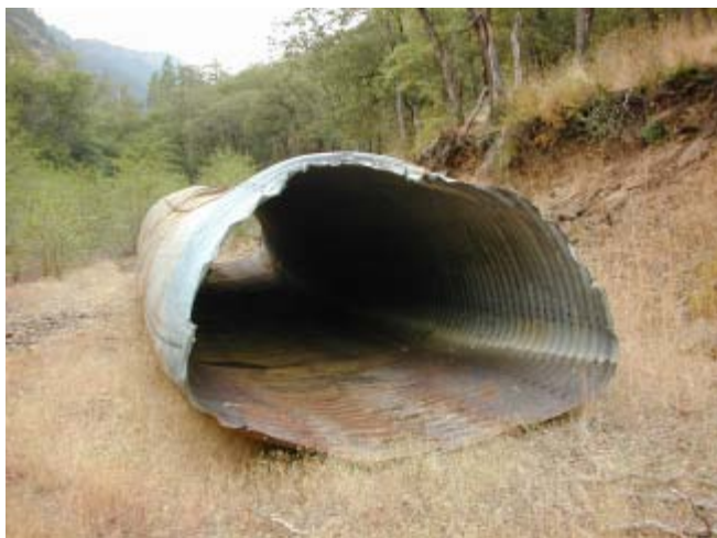
Snyder Creek 9/ 3/03 Old pipe that was removed to make way for bridge.
