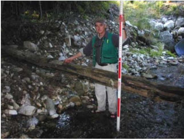
Wendover Creek 8/18/03 Kurt Beardslee with a duck bridge formed by upstream headcutting above a new culvert installation.
