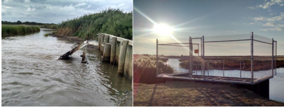
Before and after restoration of a water control structure in Little Creek Wildlife area, DE.
