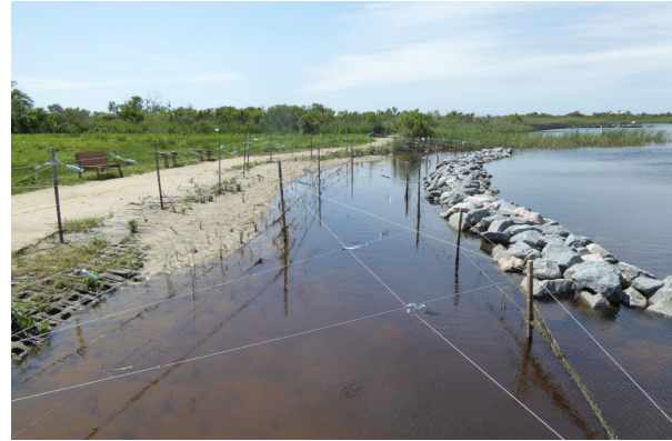
Back Bay National Wildlife Refuge completed living shoreline construction (project final report).
