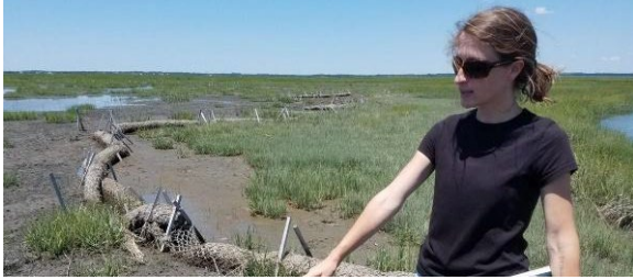
Project ecologist shows coir logs installed to contain applied dredge at New Jersey-Cape May Wetlands Wildlife area (Cape May County Herald).
