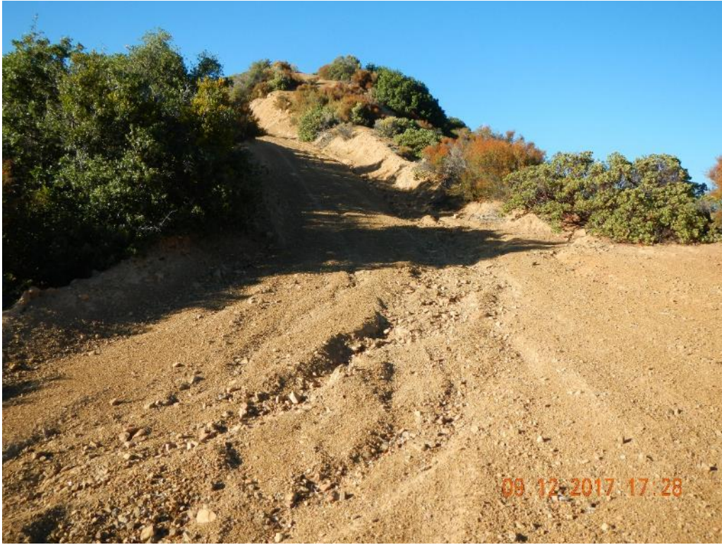
Photo 9 – Road 6N03 eroded road surface Eroded road surfaces on 6N03 (top and bottom).
