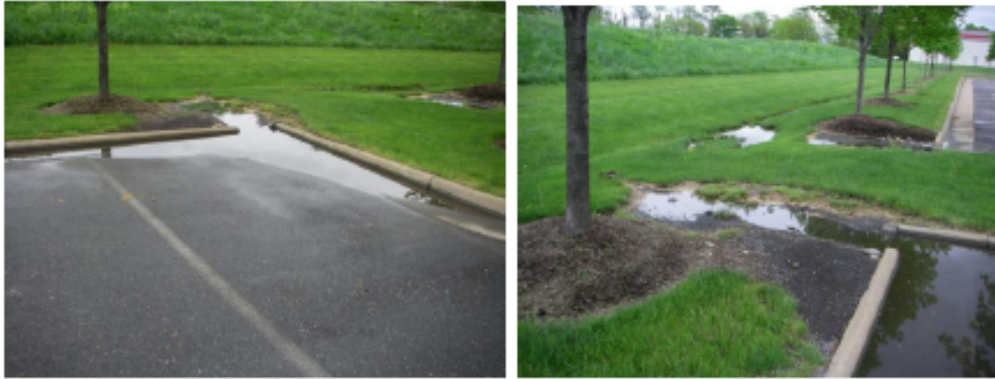
Ponding at curb cuts
