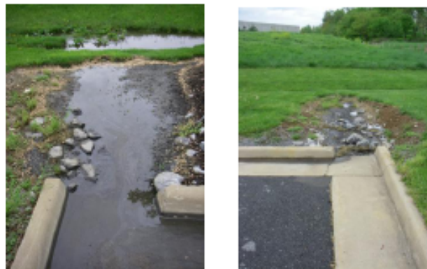
Erosion at curb cuts
