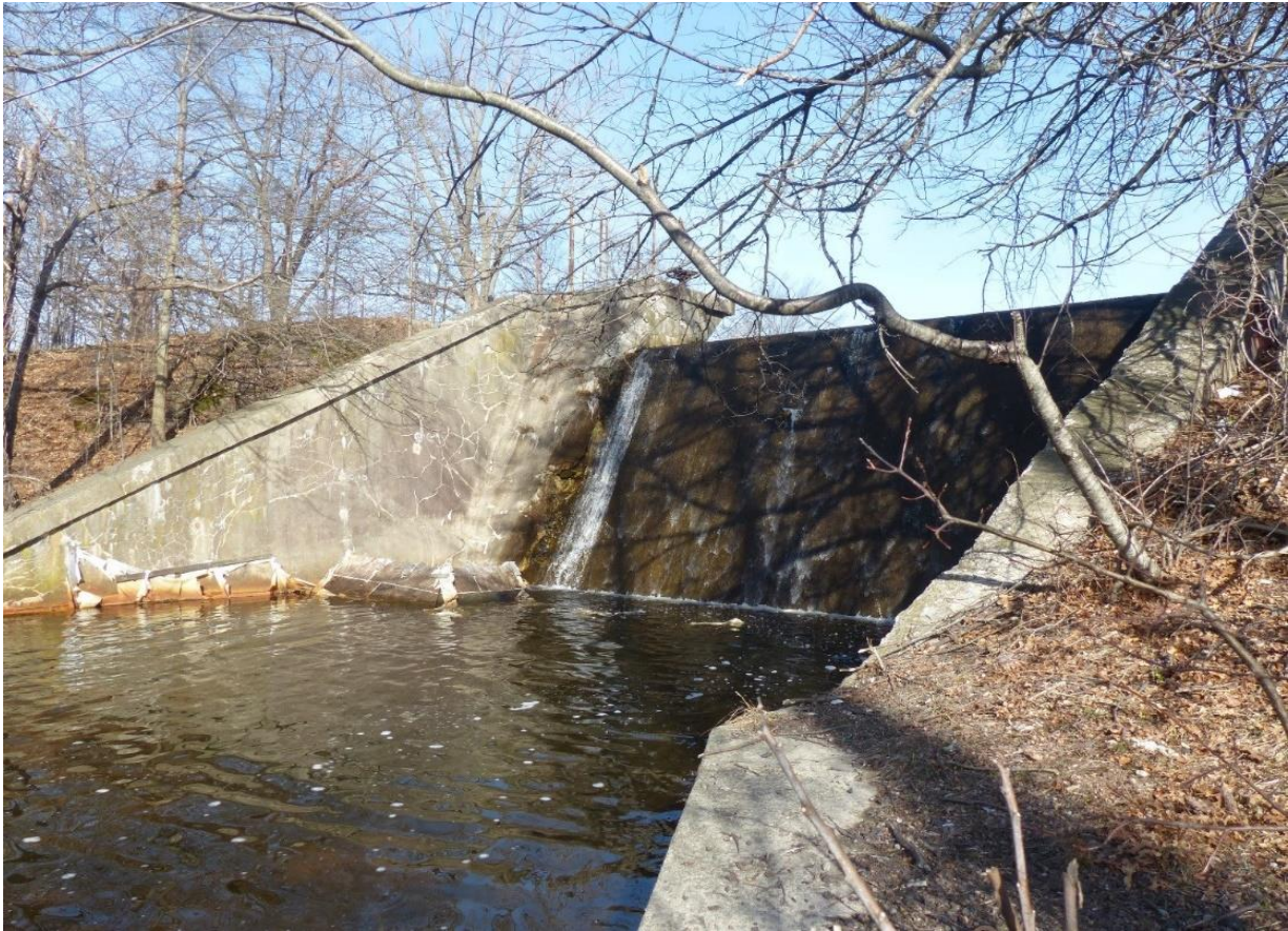
Figure CS1-1. Photo of Canada Pond Dam showing cracks and other signs of age.
