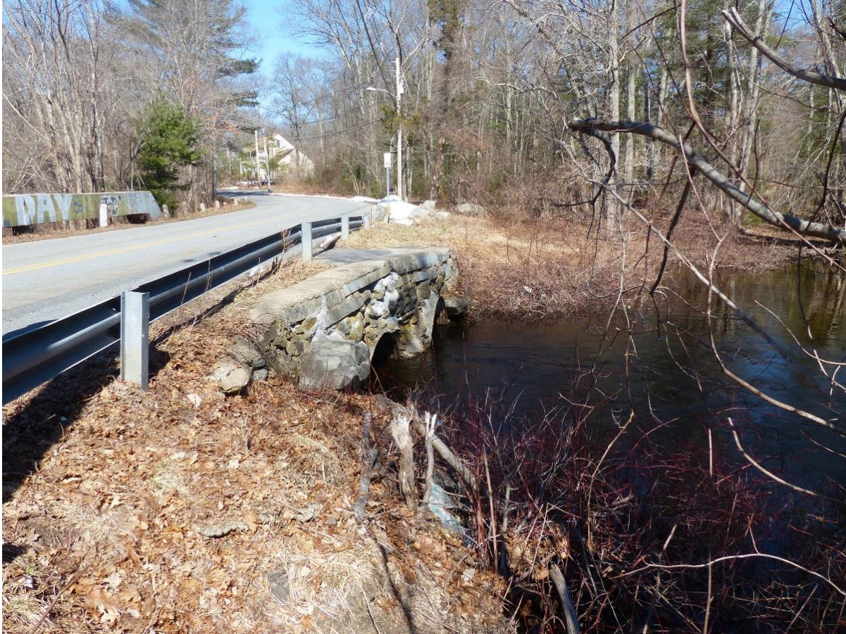
Figure CS3-1. Photo showing under-sized culvert on the Wading River, Norton, MA.
