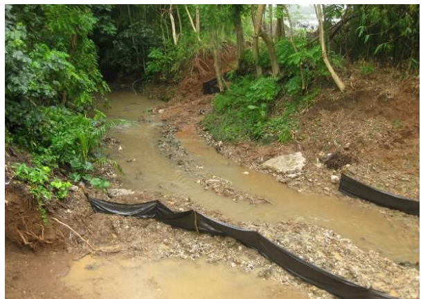
During wet weather, you may observe tremendous sediment plumes from areas with inadequate vegetation or construction activities.
