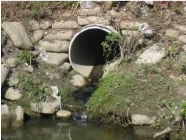
Evaluate dry weather flows at outfalls should for sewage or other non-stormwater flow.
